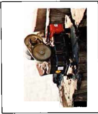
Water pressure systems
