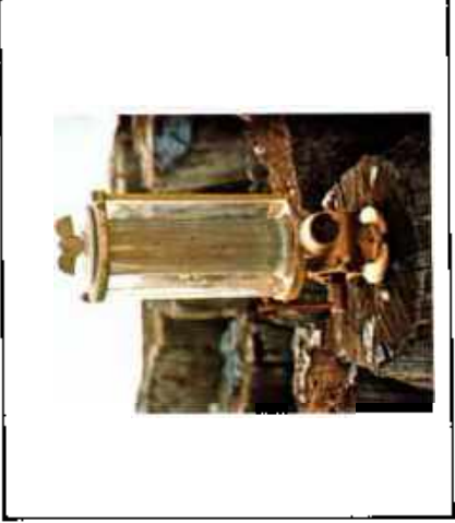
Raw water intake strainers
