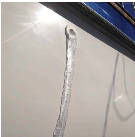
Frozen meltwater can damage thru-hull fittings.
