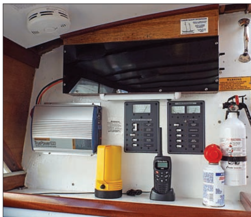
All the electrical wiring on board was replaced, and a modern electrical panel installed, as well as a 600-watt true-sine-wave inverter.
