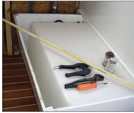
Far left —A new Par-Max 12V water pump and filter installed in the engine room is the heart of the boat's onboard freshwater system. It draws from a new 30-gal (113-l) tank installed under the aft dinette bench, left .
