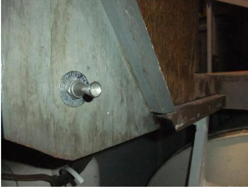
The original engine room light switch
